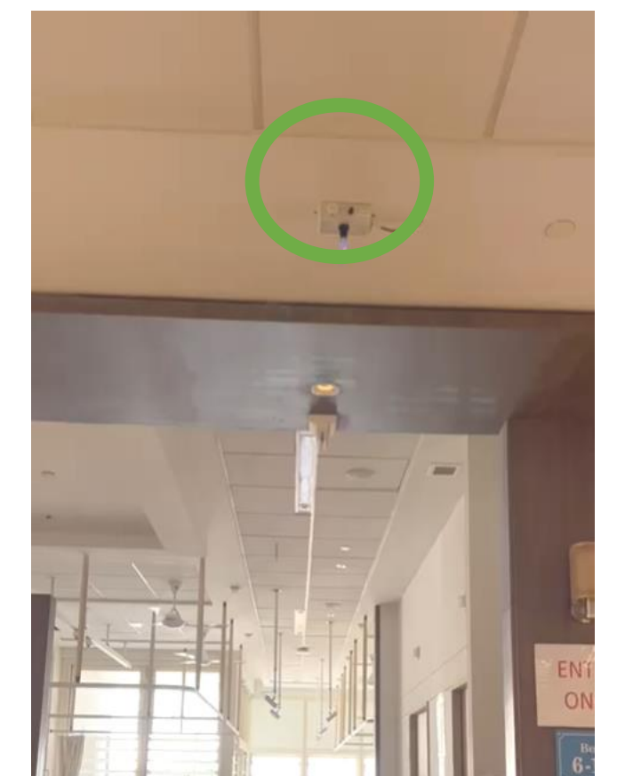
Figure 2. Alarm units on the ceiling
